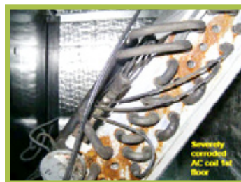
Severely corroded HVAC coil
