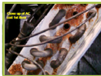
Close up of HVAC coil
