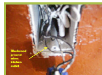
Blackened ground wires
